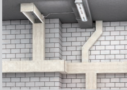
Mounted fire protection duct on wall and ceiling
