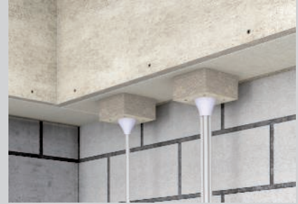
Mounted fire protection duct with cable outlets
