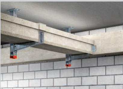
Combination of suspended fire protection duct and wall duct
